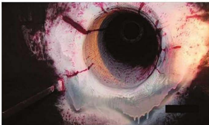
Figure 5—Cracking Observed at Quench Nozzle in a Heavy Wall Reactor Vessel
